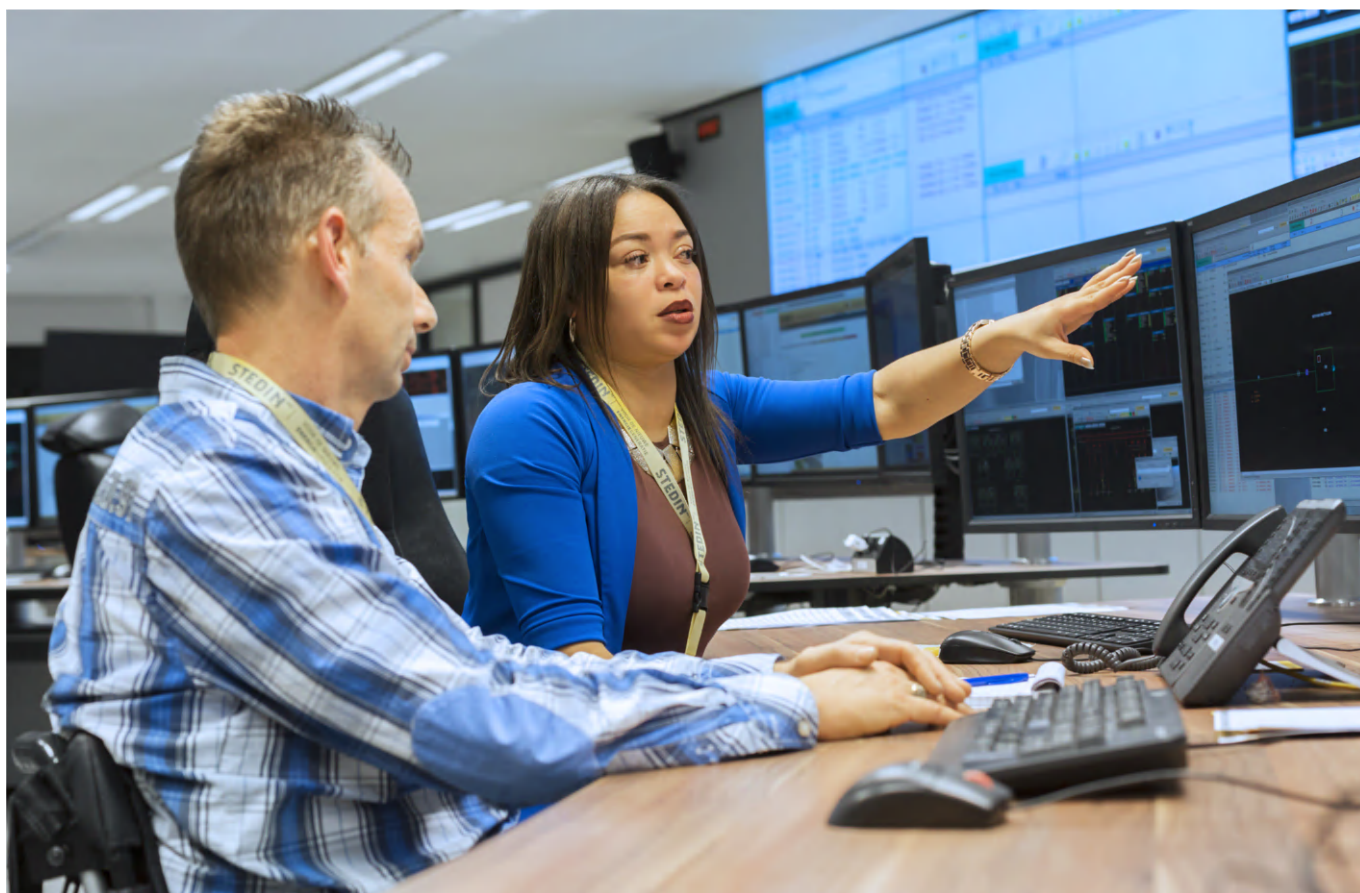
Nieuw Network Operations Center (NOC)
